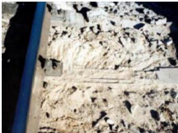
Figure 1.21 Failure of concrete tie as result of bar corrosion (Mohammadzadeh and Vahabi, 2011).
