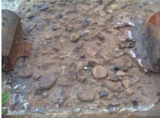
Figure 1.15 Rail-seat abrasion failure (Zeman et al., 2009)
