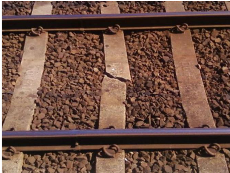
Figure 1.14 Flexural failure of PC tie due to negative bending (UK railway forums/broken tie, 2014)
