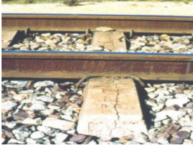
Figure 1.20 Cracking in concrete tie due to alkali aggregate reaction (Fournier et al., 2004)
