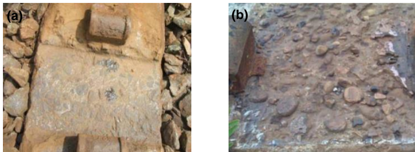
Figure 5.1 Prestressed concrete rail seat abrasion (a) Reiff et al. (2012), (b) Zeman et al. (2009)
